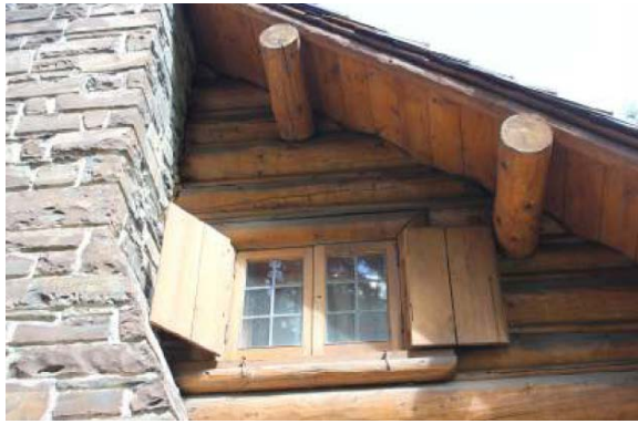
Purlins visible along the exterior roof line of the second floor of the original cabin
