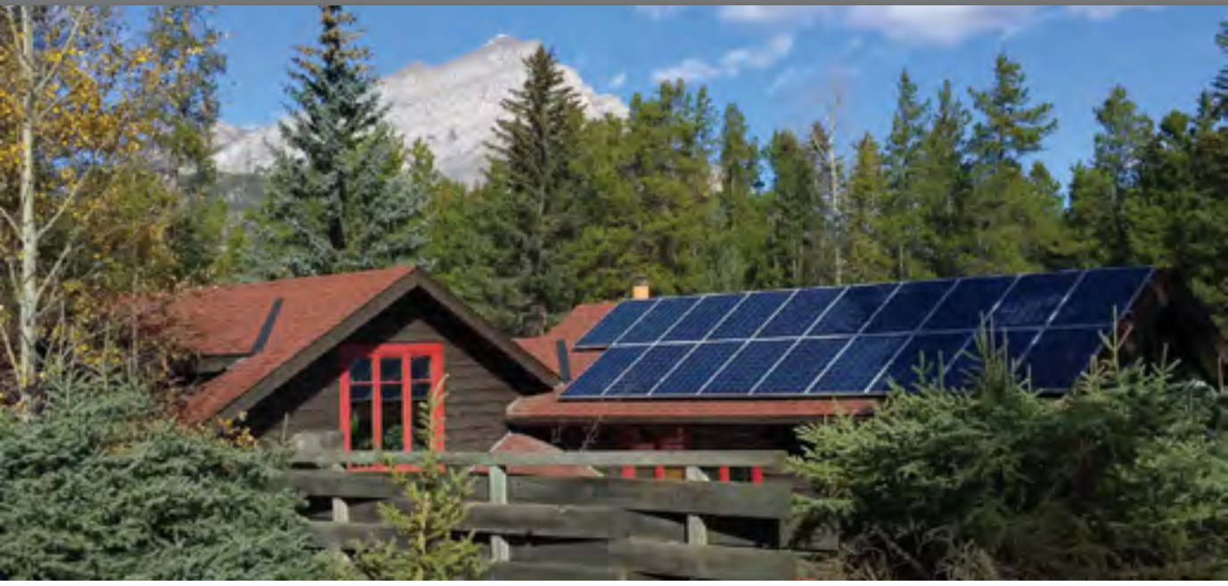
Banff Residence (131 kW)
