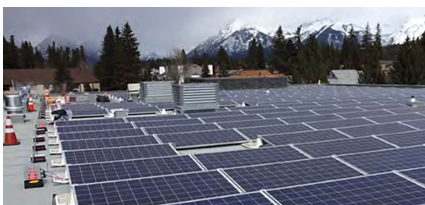
Banff Elementary School Phase I (65 kW)
